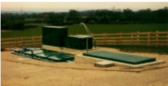
A modular HiPAF sewage treatment plant
