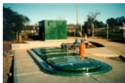
A single tank HiPAF — installed for a Water plc
