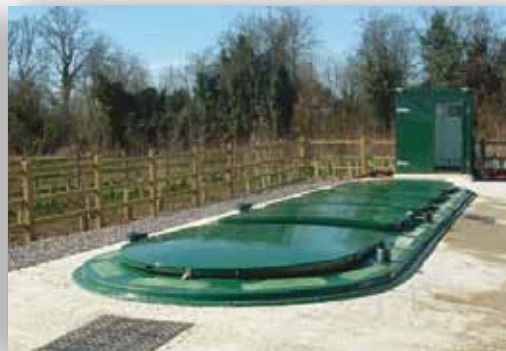
HiPAF Midi Plant with control kiosk
