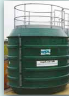
HiPAF Compact installed above ground (left)
