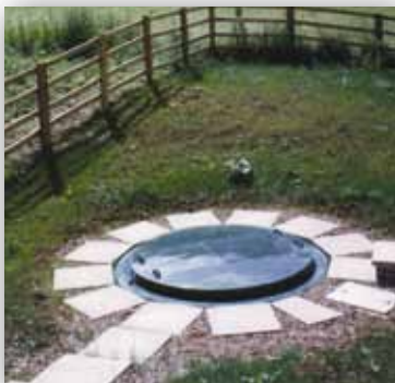
HiPAF Compact plant, below ground installation
