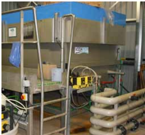
Coil pipe flocculator and DAF
