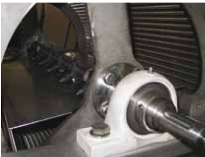
Internals of rotary drum screen
