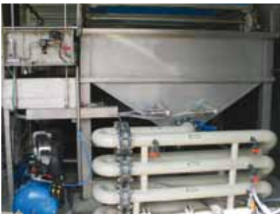
Coil pipe flocculator
